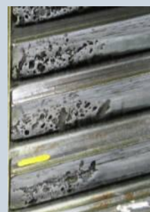
Visual inspection in Spring 2007: the old pitting was rounded off and smoothened. There are no more sharp edges and particle break outs.
